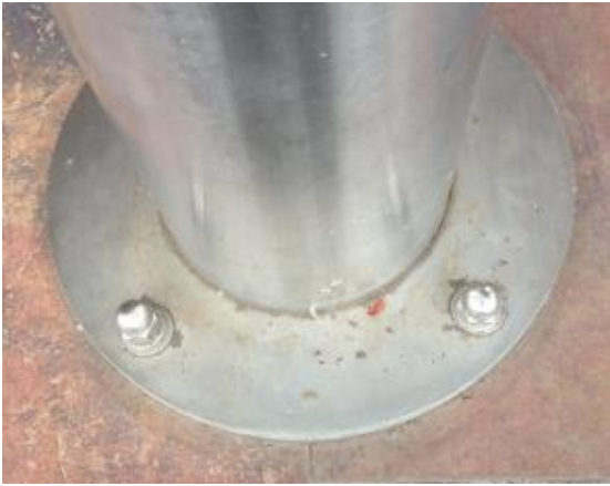
Typical stainless steel bollard with base showing crevice corrosion
