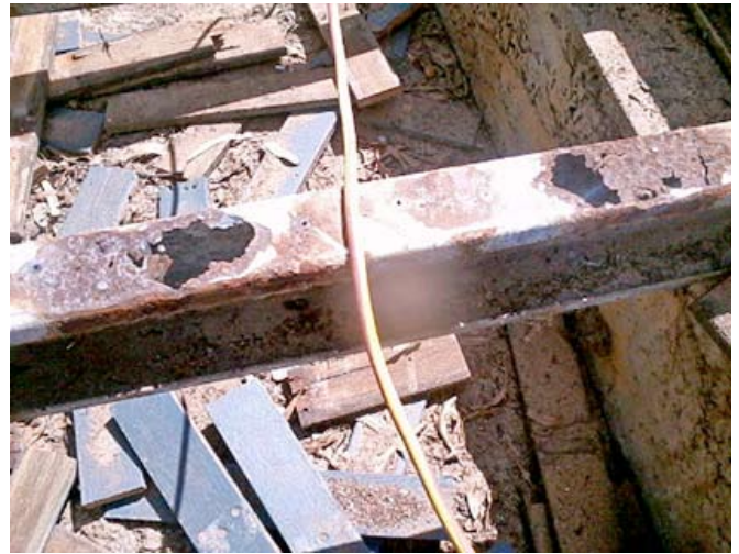
Corroding C section joists Image courtesy of Contrast Constructions
