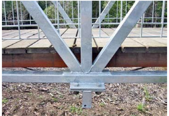
Unsuitable gauge steel needed additional plate to take the load as well as climbing toe holds on handrail
