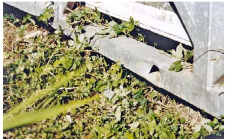
Unsuitable gauge steel damaged by mower
