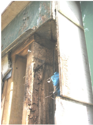
The corner supporting studs are totally missing at the top
